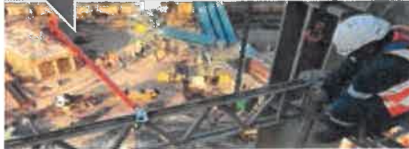
SGB Cape: QuikDeck platform being assembled in the air by a specially trained Waco employee.
