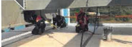
SGB Cape: Vulindlela Project where the QuikDeck team complete the QuikDeck Suspended Access System.
