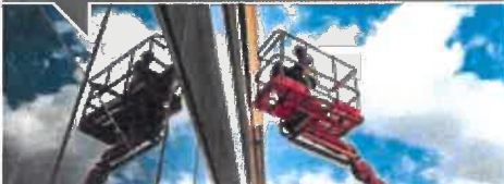
SkyJacks: Working safely at heights during construction of Barloworld Equipment's new head office, Isando, South Africa.
